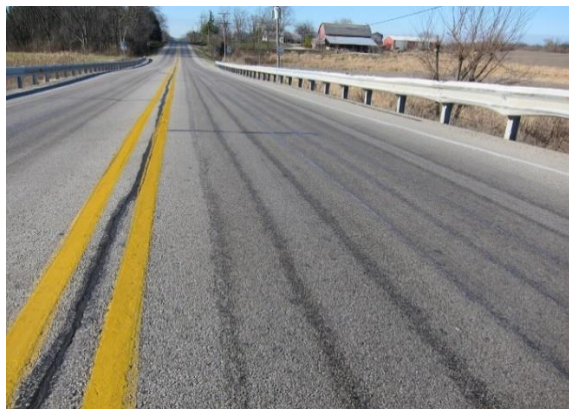
Striping on road from liquid “anti-icing” application
