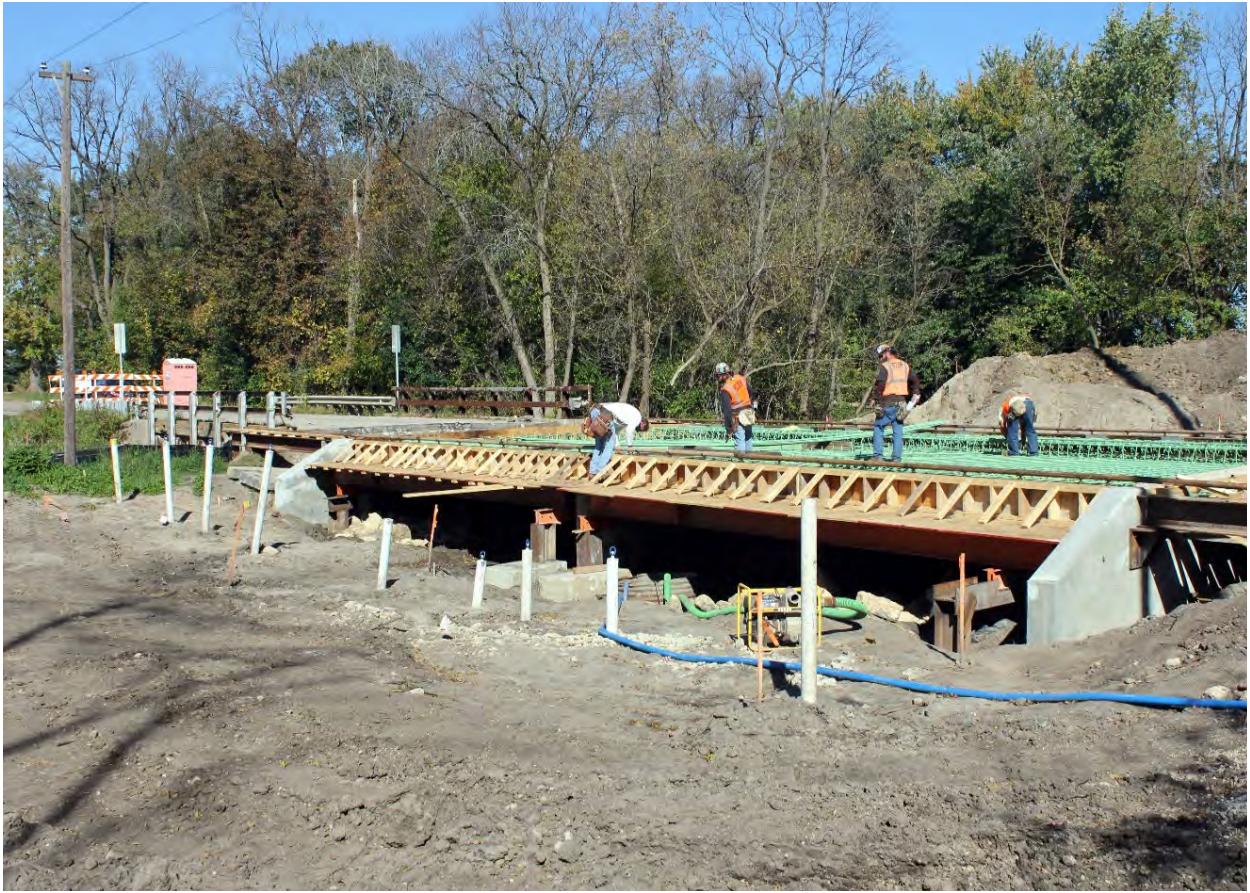
The bridge was completed during Stage 1 "in the dry" to minimize channel impacts.
