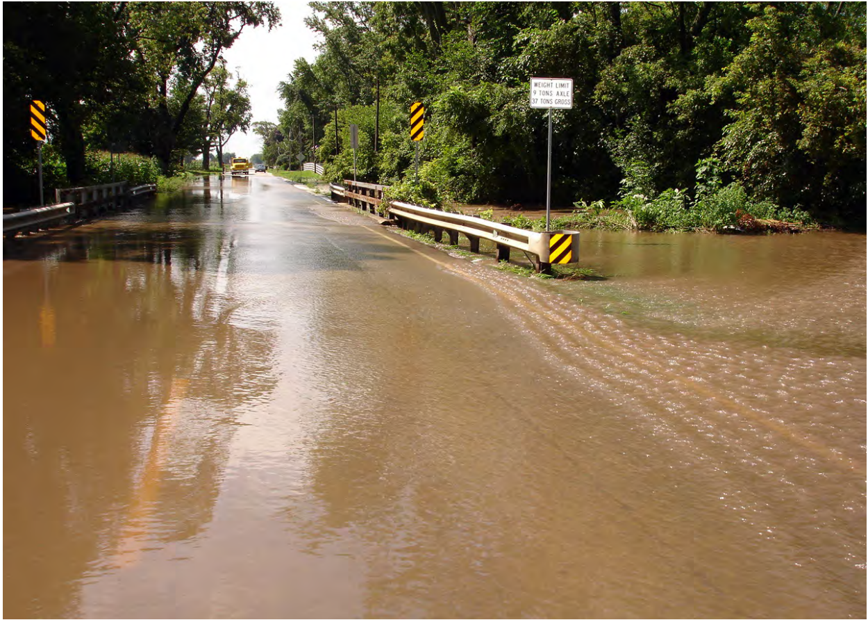
The existing bridge experienced overtopping during the 10 year rain event.
