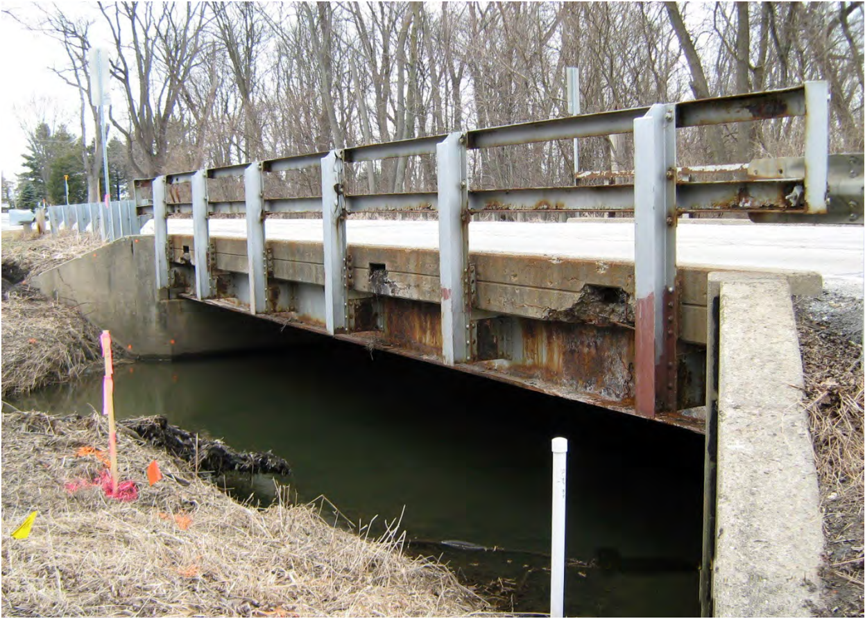
The existing bridge had experienced significant deterioration and received a sufficiency rating of 25.6.
