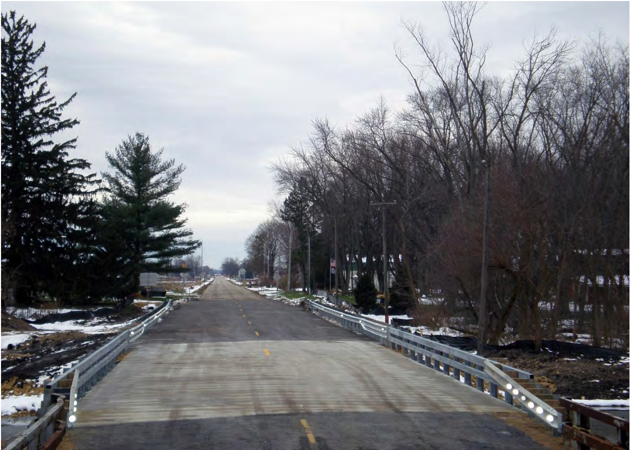
A temporary guardrail transition design allowed for the roadway to be opened safely during winter shutdown.
