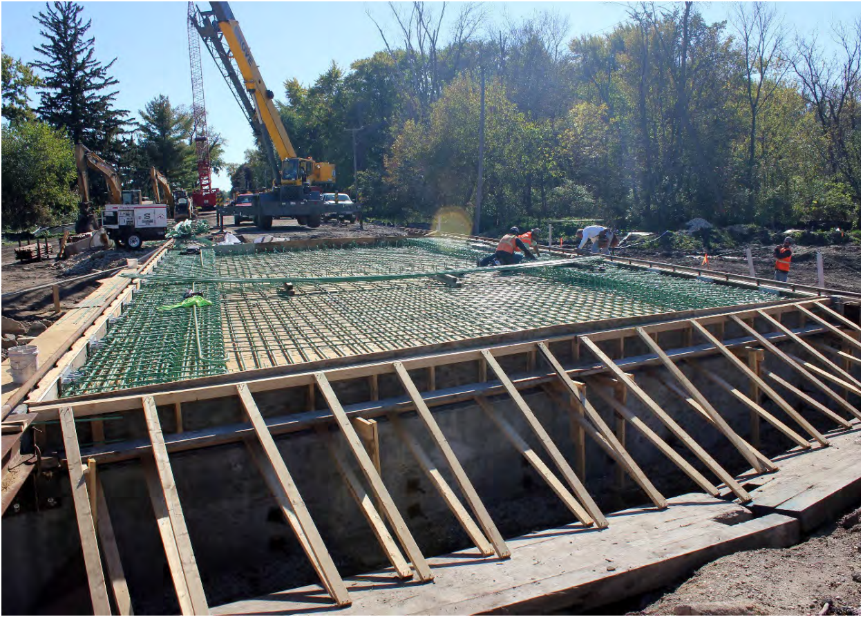
Deck framing and reinforcement, as the slab bridge minimized the depth of the structure and maximized the bridge opening.
