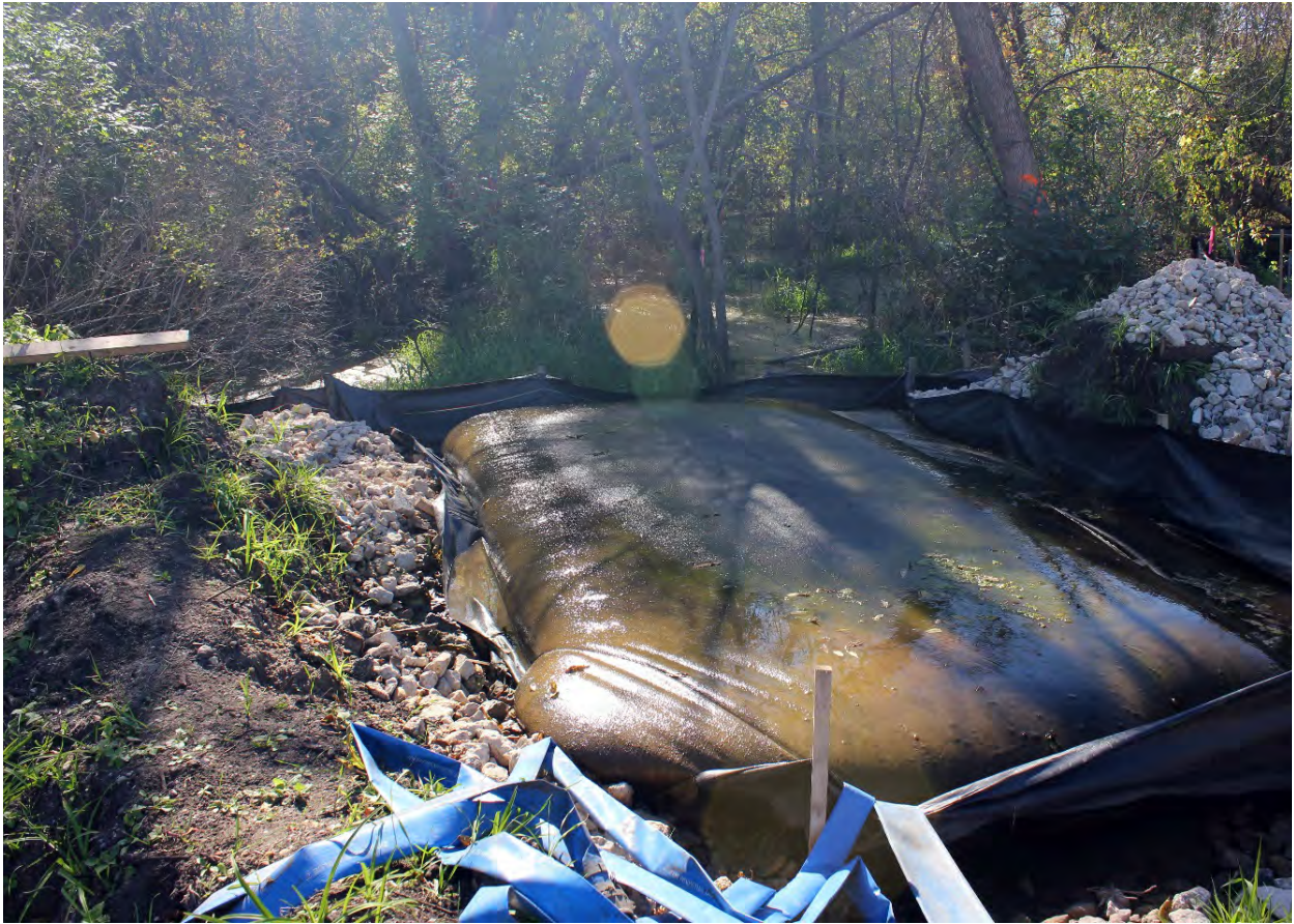
Sediment bags were one of the many BMPs used on site to minimize erosion.
