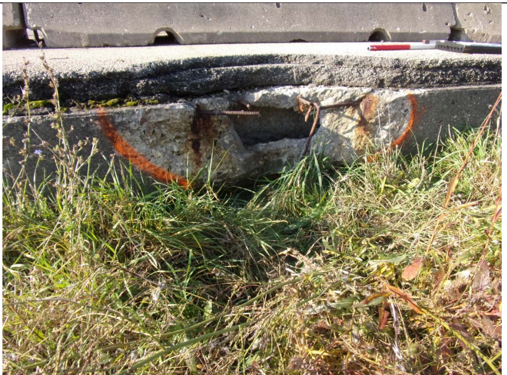
Photo 7 Viewing collision damage to outer beams.
