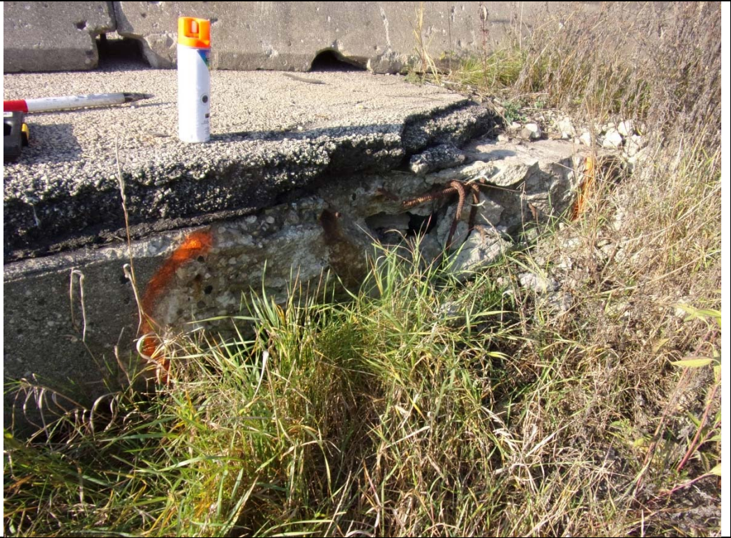
Photo 8 Viewing collision damage to outer beams.
