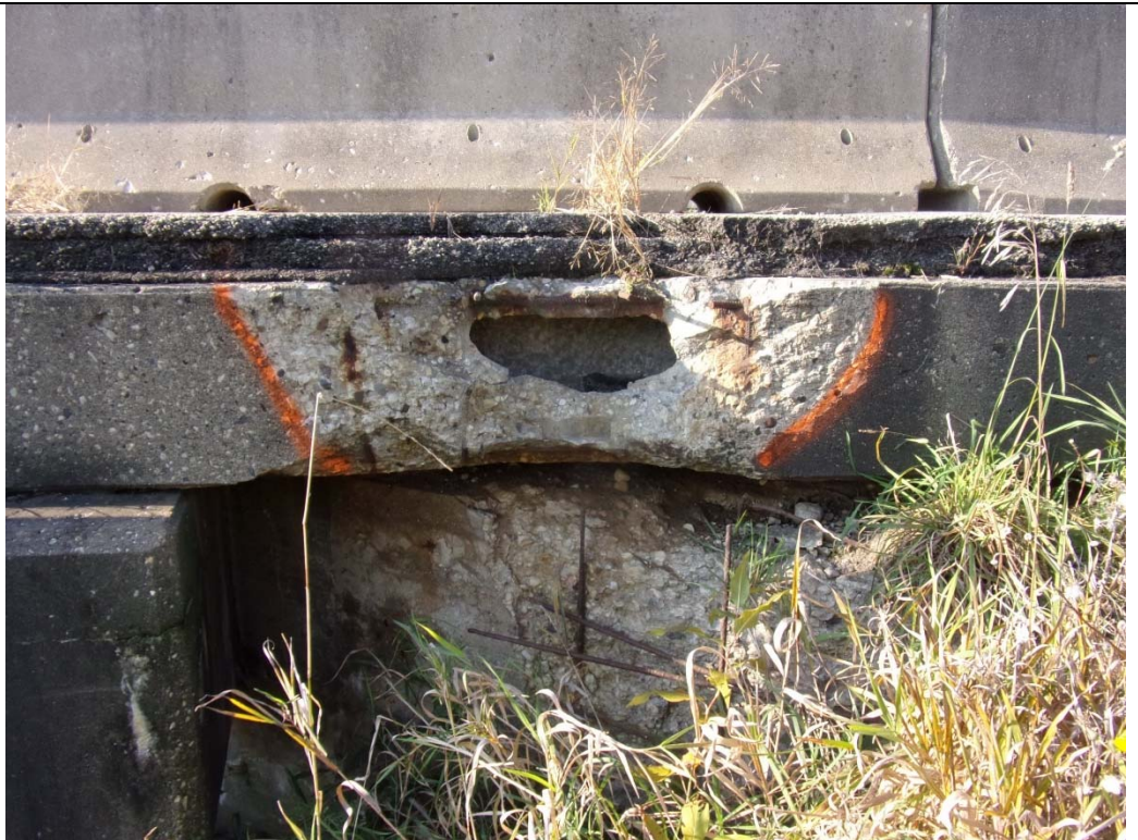
Photo 6 Viewing collision damage to outer beams.
