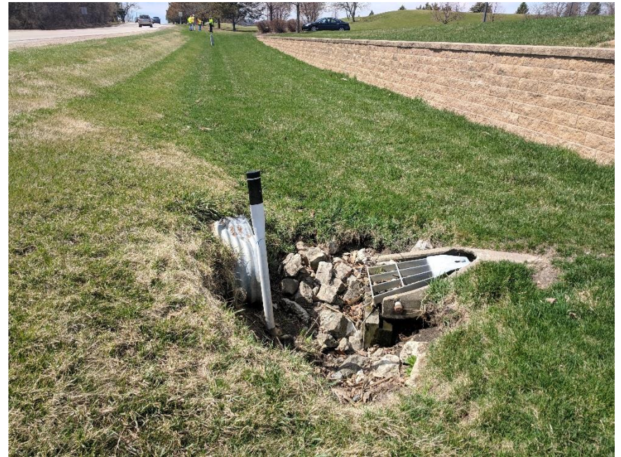
Ackman Rd, between Albrecht Rd & Redtail Dr Non-traversable culvert end section with steep grades and eroded ground
