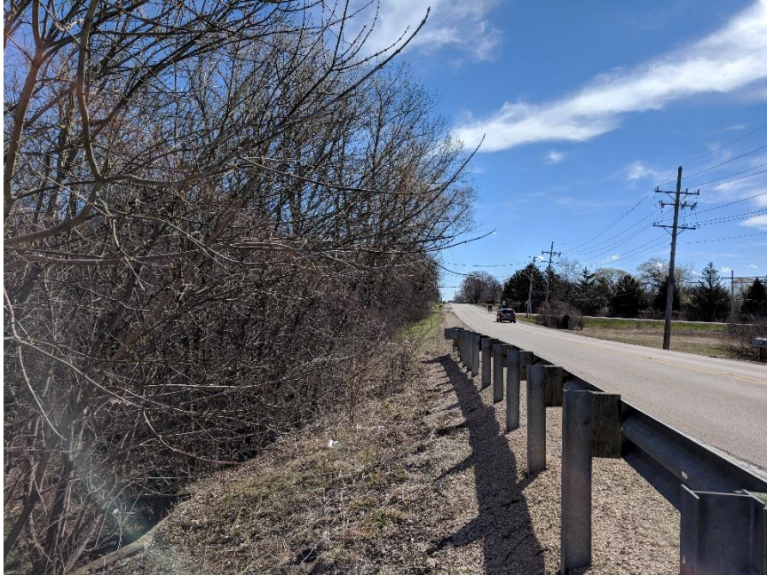
Ackman Rd, between Redtail Dr & Swanson Rd Non-recoverable, unprotected foreslope on approach to culvert hazard
