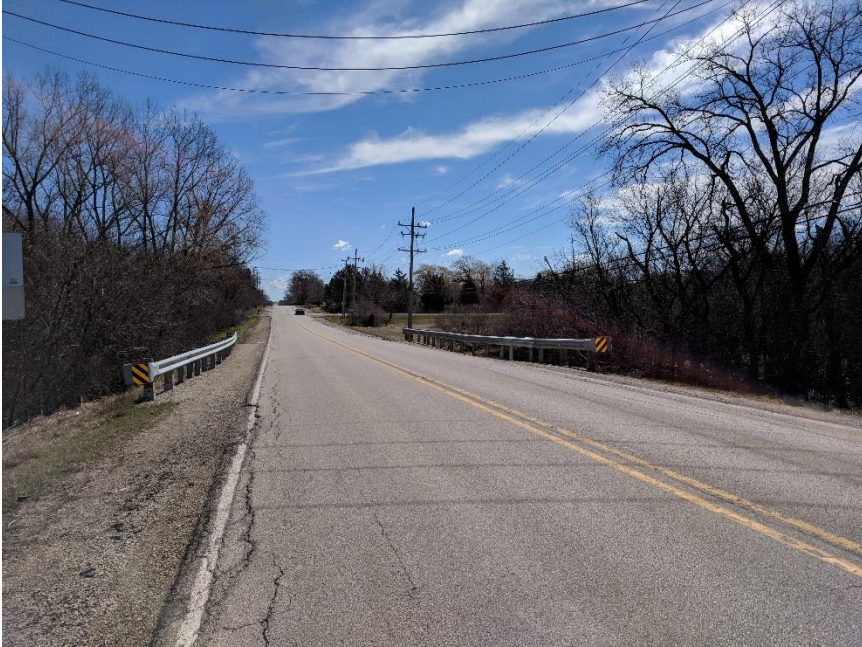
Ackman Rd, between Redtail Dr & Swanson Rd Guardrail limits do not cover length of need for culvert and foreslope hazards.
