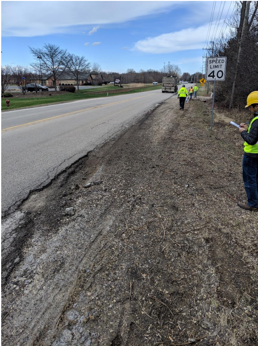
Ackman Rd, between Albrecht Rd & Redtail Dr Damaged EOP
