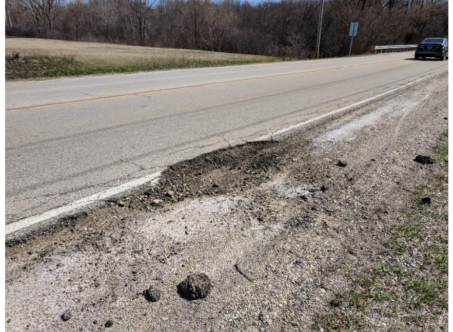
Redtail Dr & Ackman Rd Edge of pavement damaged
