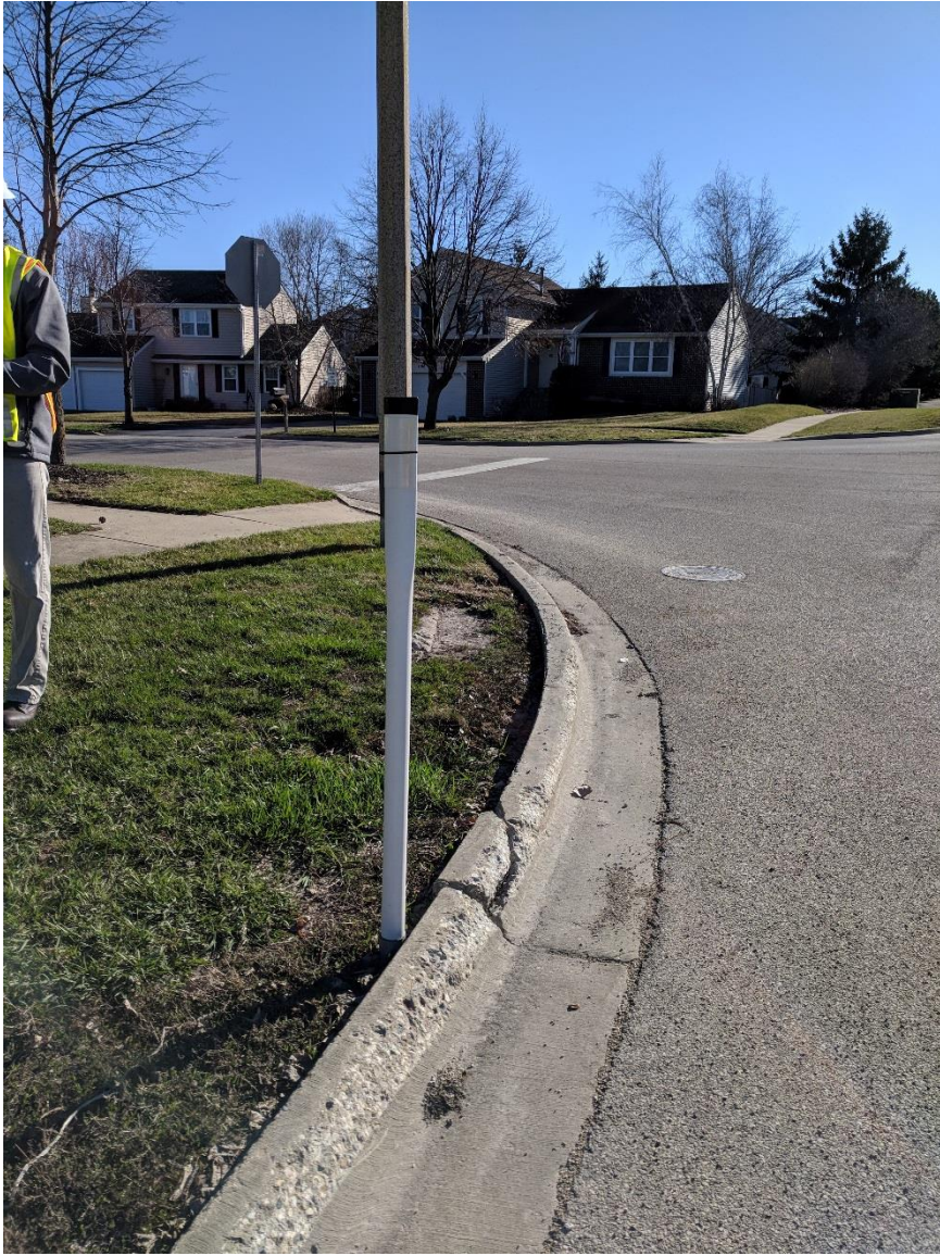
Crimson Dr & Ackman Rd Broken curb at NW corner radius
