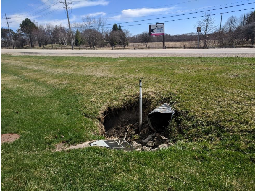
Ackman Rd, between Albrecht Rd & Redtail Dr Non-traversable culvert end section with steep grades and eroded ground
