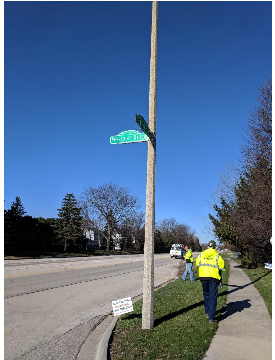
Crimson Dr & Ackman Rd Non-breakaway light pole in clear zone
